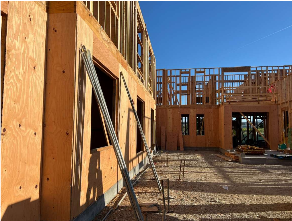
Exterior plywood sheathing installed on the eastern elevation of the first floor.
