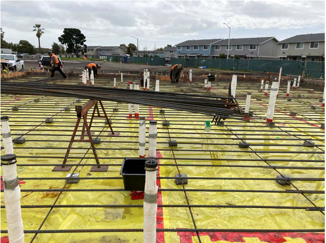
The long metal poles are rebar to reinforce the concrete for the building foundation. The white pipes are for underground plumbing.
